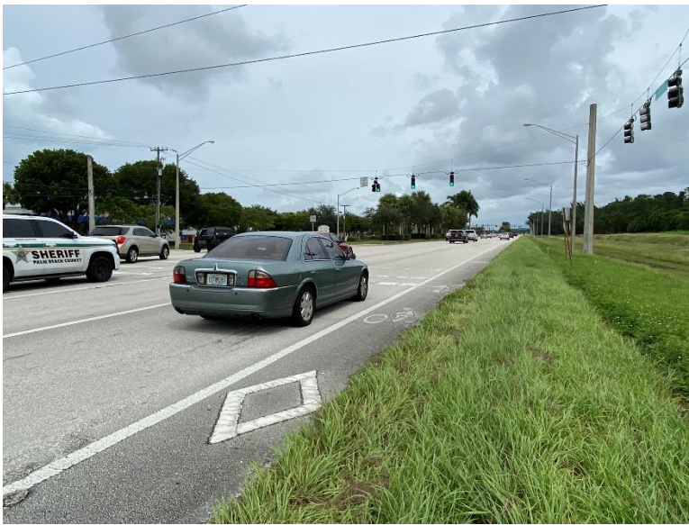
There is no sidewalk on the east side of SR-7 and the bicycle lane is encroached by grass.
