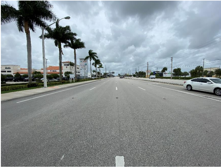
Eastbound four (4) through lanes of Okeechobee Blvd west of I-95 looking west.
