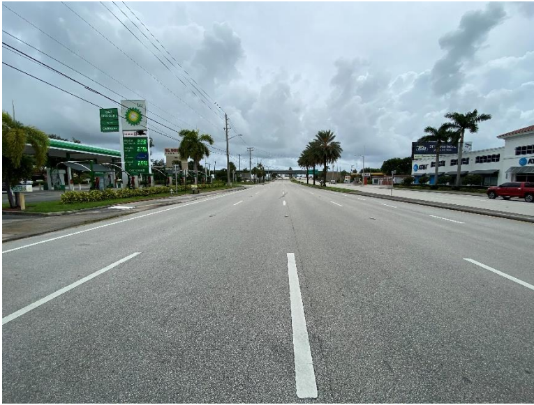
Westbound four (4) through lanes of Okeechobee Blvd west of I-95 looking east.
