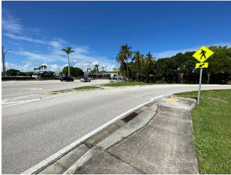
The crosswalk on the north side of Okeechobee Blvd across the Australian Avenue northbound on-ramp looking west.
