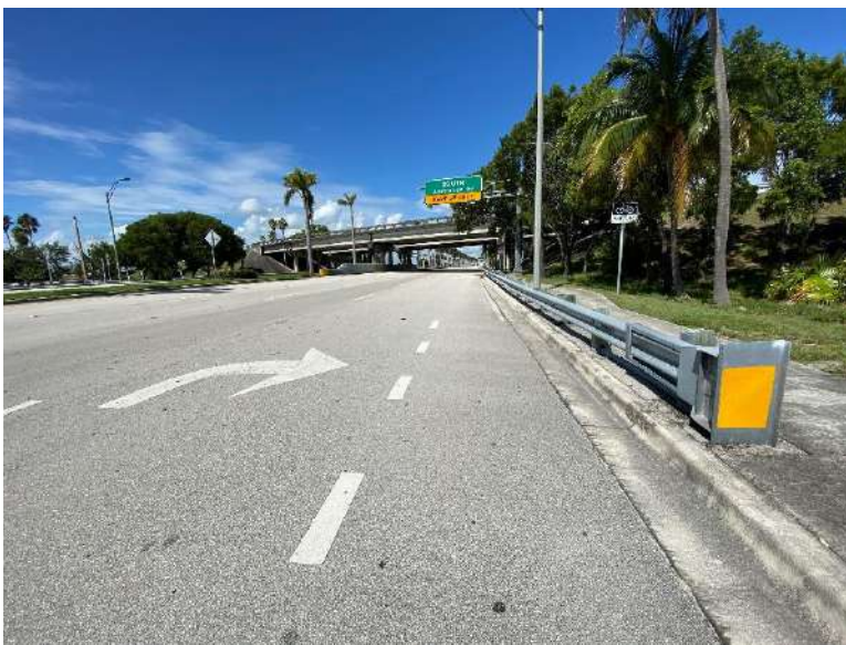
The westbound direction of Okeechobee Blvd includes an unbuffered bicycle lane transition due to the cloverleaf on-ramp to southbound Australian Avenue.
