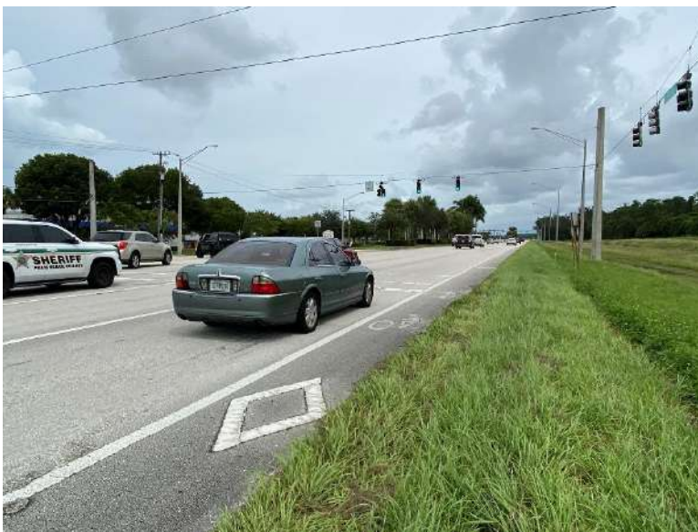
There is no sidewalk on the east side of SR-7 and the bicycle lane is encroached by grass.
